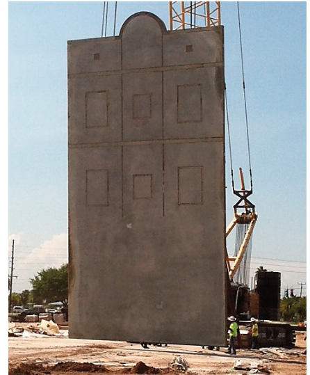
Steelmaster Industries is known for its expertise in concrete tilt-wall construction, including insulated tilt-walls.
